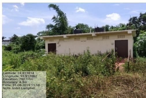
Locked Public Toilet, Lamphel CC, with no approach road to access the toilet
